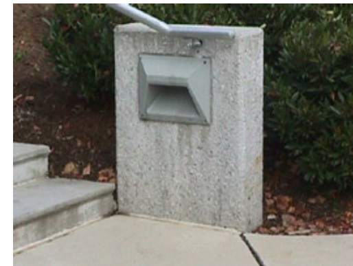
LIGHT FIXTURE (EXHIBIT E)
